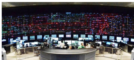
NYISO control room Source: NYS Smart Grid Consortium
