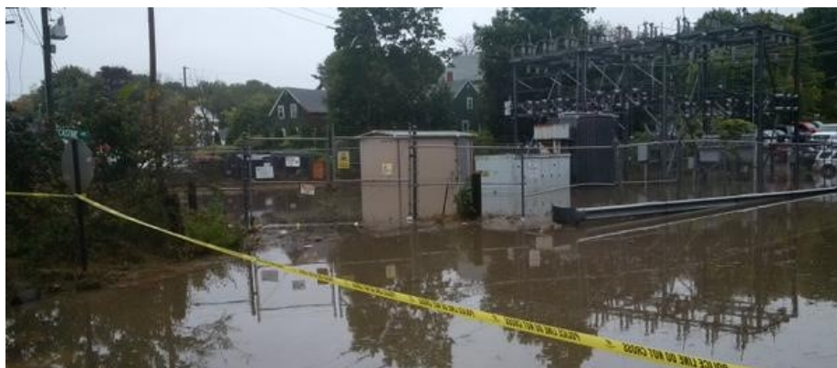
Storms flooded Central Maine Power's substation in Bath in September 2015. Source: Central Maine Power
